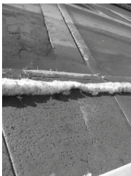
Figure 5: Expansion Joint & Normal Concrete Sidewalk Scaling
