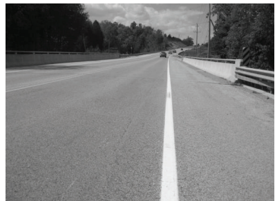
Figure 3: Longitudinal Cold Joint in Asphalt
