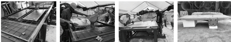
Figure 2: Different stages of the keystone construction at Bieton field office in Medellín (Colombia).
