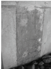
Figure 2: Cracks in Vertical Connection (non-UHPC)
