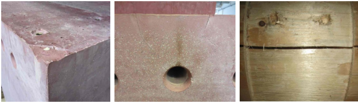
Fig. 13. Damage to the upper corner of N-block (left), cracks above the holes (middle) and damage to a tenon hole in one of the logs after the end of the campaign. (photos by S. Schuster)
