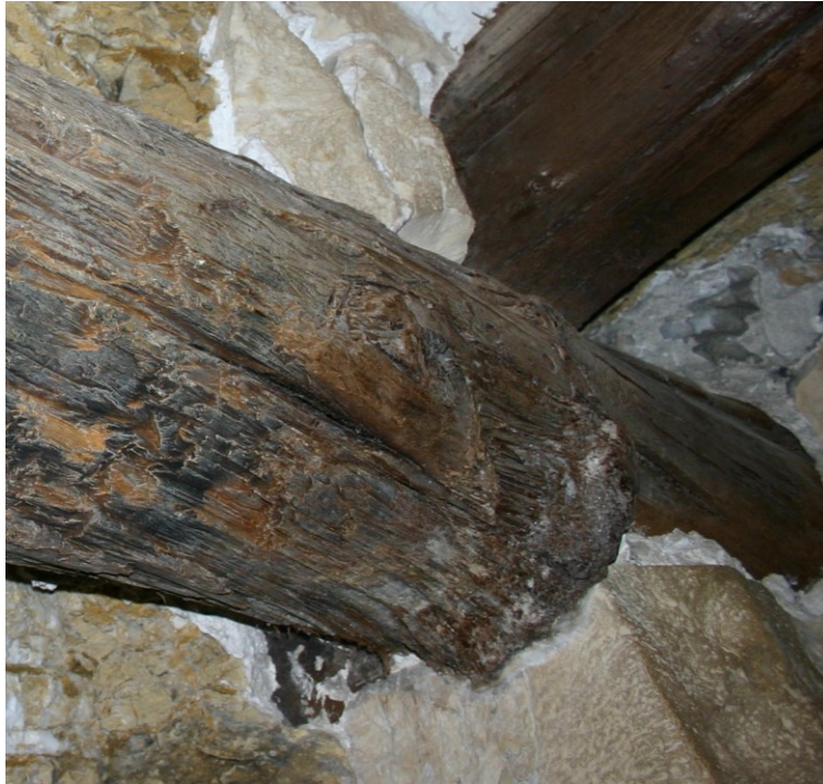
Fig. 8. Damage on a construction log in the Meidum Pyramid caused by a moving rope (photo by U. E. Dorka)
