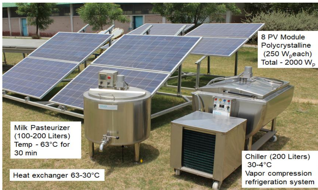
Figure 4.3: Complete solar chiller unit installed at Solar Campus, UAF
