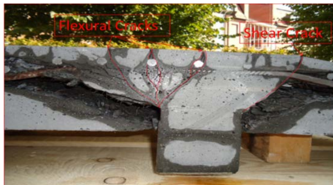
Fig. 4.4: Flexural and shear cracks
