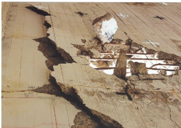
Fig. 1.3: Punching shear failure in a bridge deck [16]
