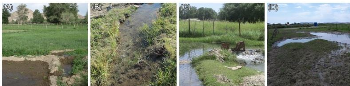
Figure 5. Reasons for irrigation losses and necessity of canal maintenance: (A) practiced surface irrigation, (B) high occurrence of sedimentation and vegetation within the canal, (C) dilapidated canal junction and (D) leakage in canal walls in Bulgan sum , Mongolia, 2013.
